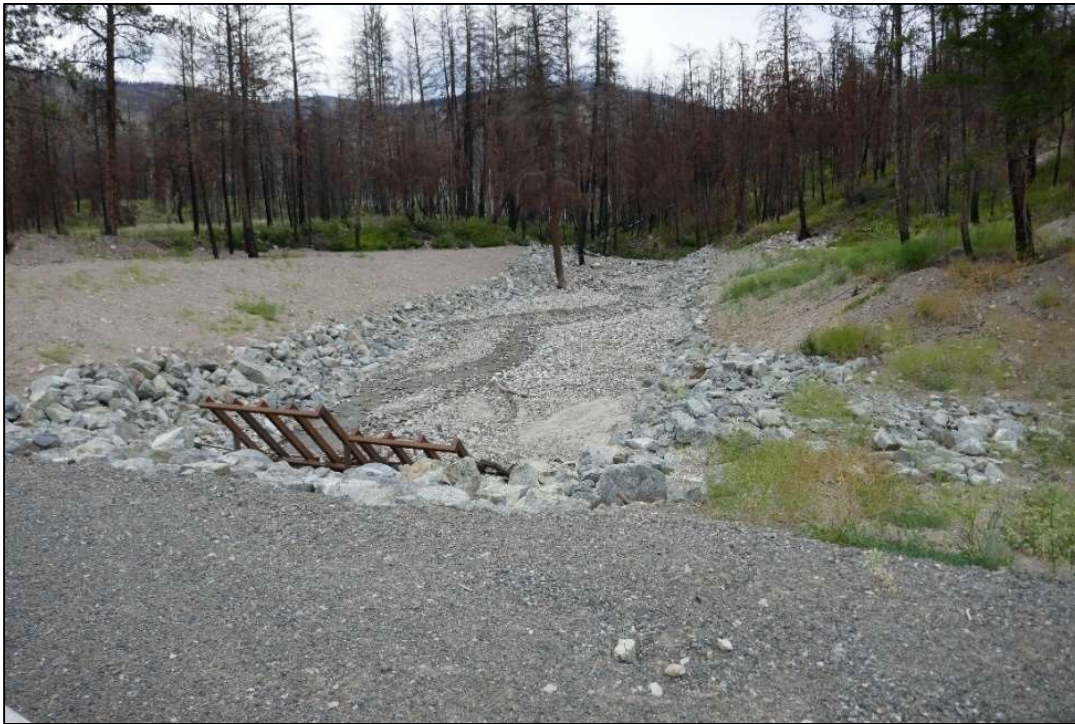
Photo 26: Construction of a wide channel through an armoured catch basin with a trash rack at the culvert inlet, such as shown in this image, may be a suitable solution at the highway crossing of Aylwin Creek.
