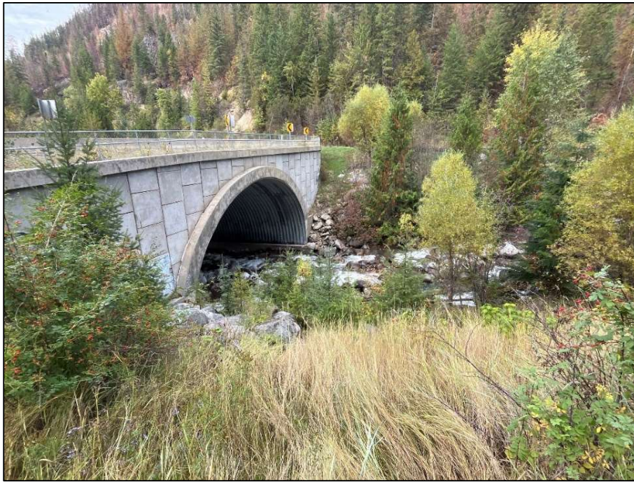
Photo 17: View of the inlet of the large arch culvert on Enterprise Creek at the Highway crossing (Field Observation Site K43).
