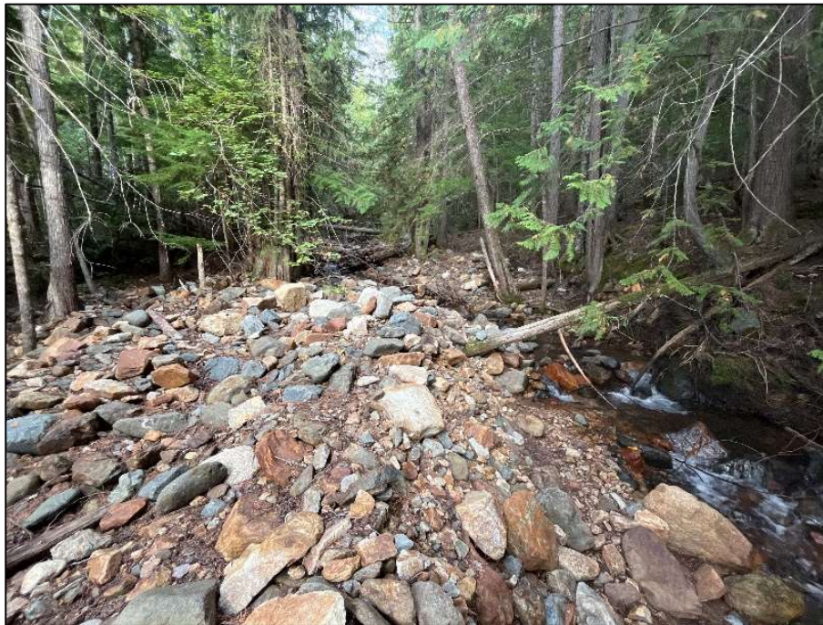
Photo 9: View upstream along Aylwin Creek immediately upstream from the Highway crossing (a 2000 mm steel plate culvert). The creek is filled with coarse cobble and boulder gravels and large wood pieces. Streamflow is diverting around the elevated sediment accumulations (aggradation).
