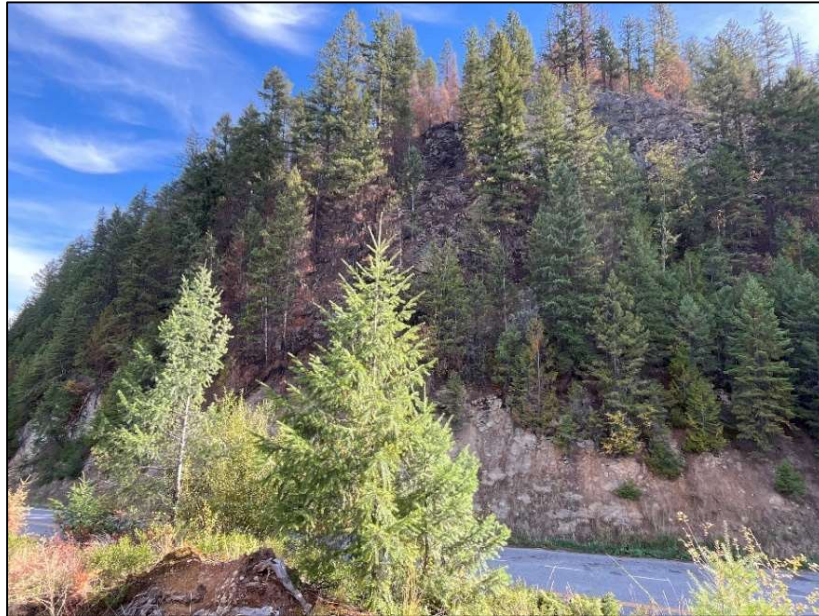
Photo 27: View of exposed rock above the Highway near the Slokan Lake View Point (Field Observation Site K28). The upper slope has a few burned patches from which vegetation cover has been removed and is the likely source of the rock that fell during the summer.
